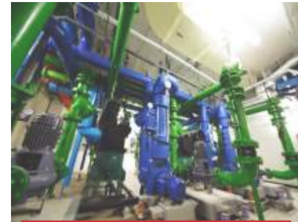
Chiller plant room
