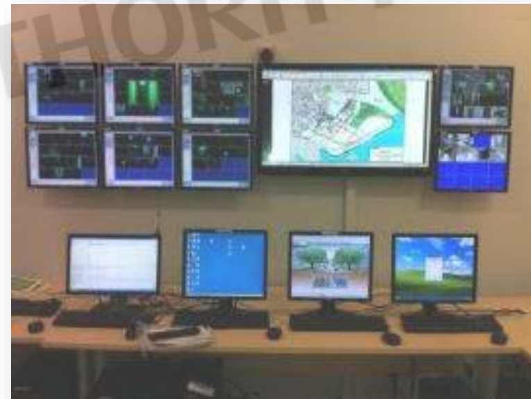
CCTV Camera and Monitor
