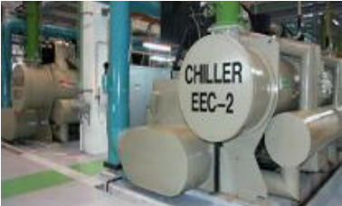
Highly Efficient DCS Plant Optimal Utilization of chiller system
