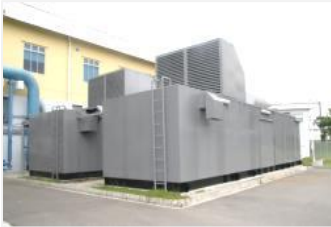
Backup Diesel Generators
