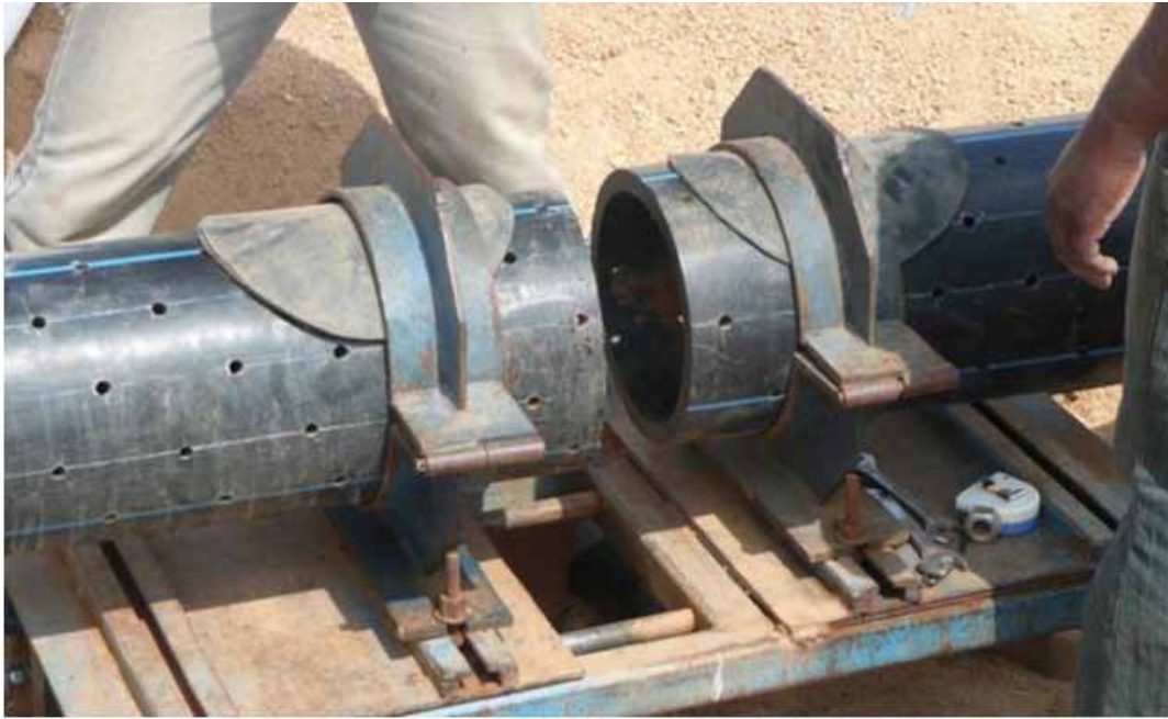
Figure 4.19: Proper Holed Leachate Pipes 24
