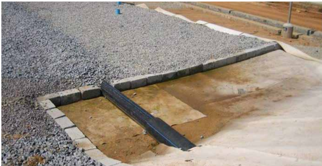
Figure 4.15: Test Field with all Sealing Components 19
