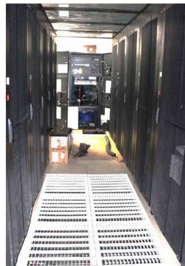
Figure 11 Server Room, Source-Author
