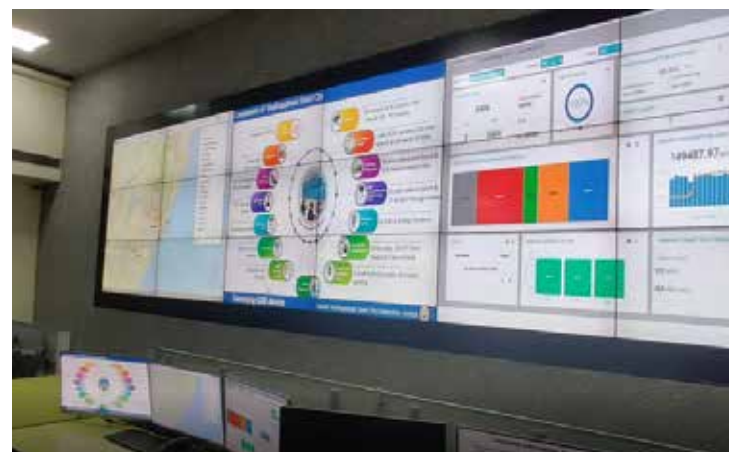
Plate 05: Dashboard with various sub-systems in ICCC
