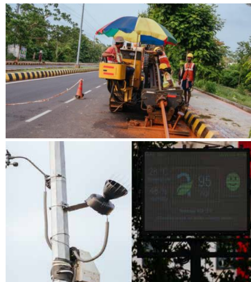
Figure- 21: Laying of Fibre Optics Network (above) and Environmental Monitoring Systems (below) (BSCL, 2022).
