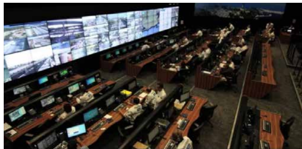
Figure-2: Rio Operations Centre, Rio de Janeiro Source: (MoHUA, 2018)
