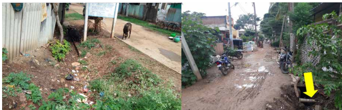
Image 2: Improper disposal point and irregular section of drain and silt deposition.
