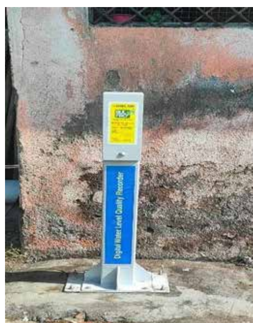
Piezometer installed at Sant Kabir School Source - Author
