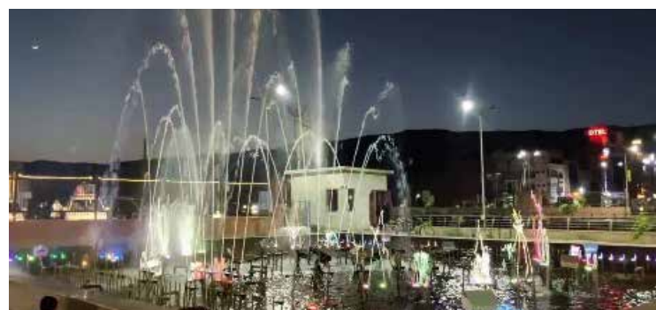
Figure-3: New Muscial fountain installed
