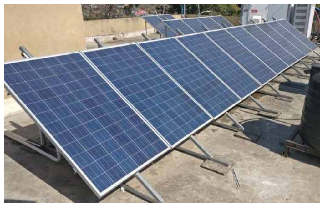
Figure-6: Solar PV module on the rooftop of Municipal Corporation building of Dharamshala Source: Rooftop Solar detailed project report
