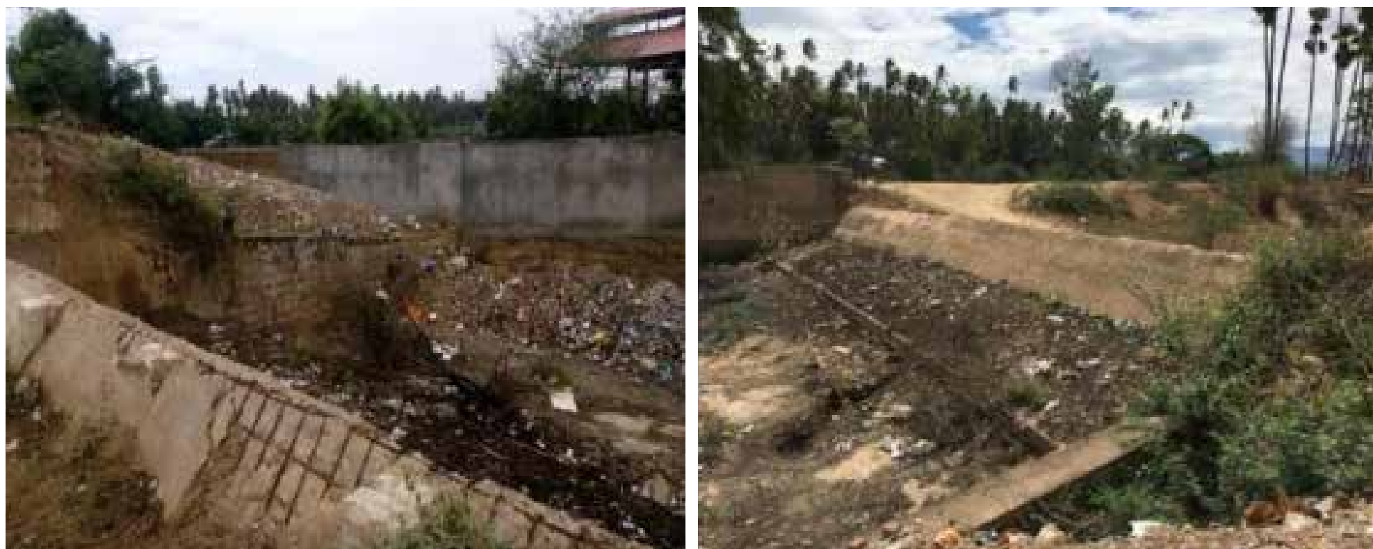
Figure 6 - Damaged wall Source: Author
