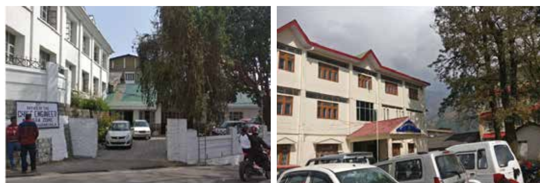
Figure 14. Solar PV system installed on buildings in phase-II Source: Rooftop Solar detailed project report
