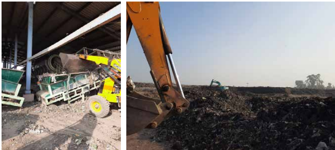
Figure 8 - Images of the processing plant and excavation of legacy waste mining (Source - Author)
