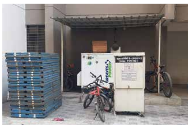
Image 4: Power Supply Units
