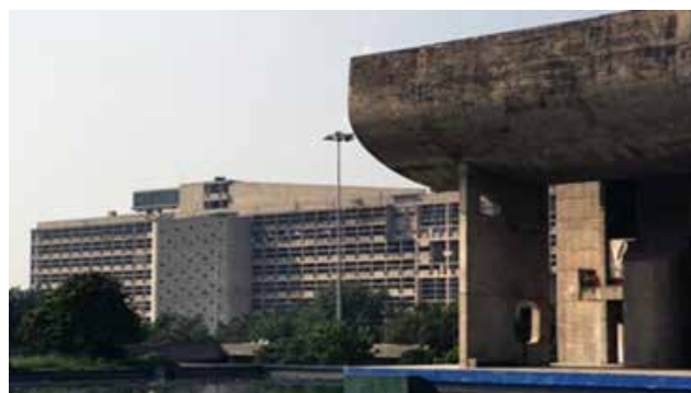
Figure 2.2: The weathering of concrete in the High Court Building; Source: Chandigarh Smart City Limited
