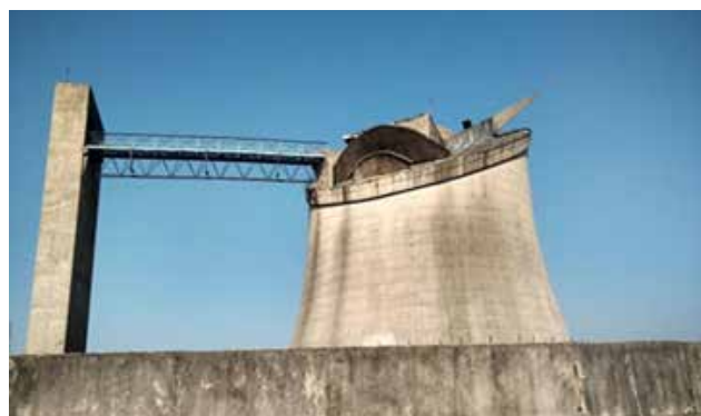
Figure 2.1: The condition of the Secretariat before restoration was undertaken Source: Chandigarh Smart City Limited
