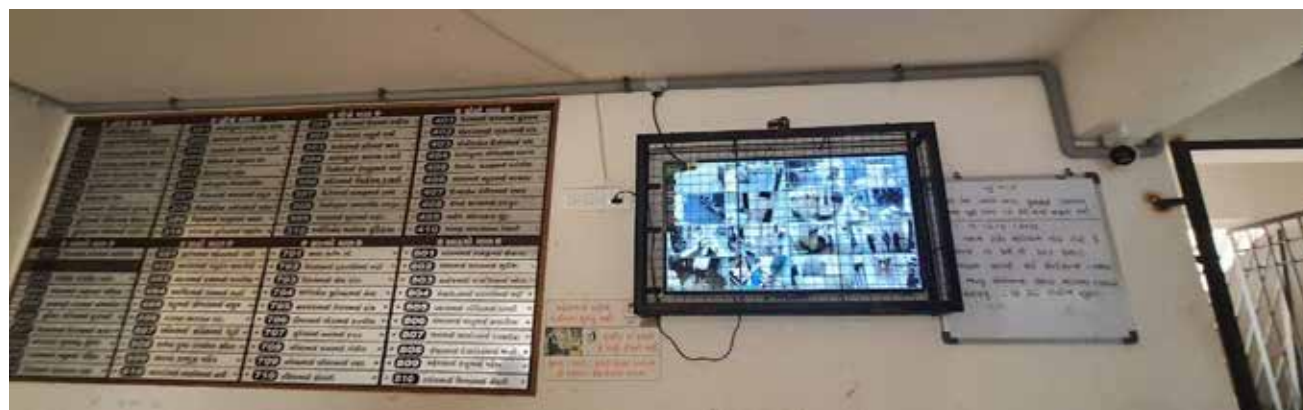
Image 9: Boards with campus name, owner name ad flat no and security monitors at the entrance of every building
