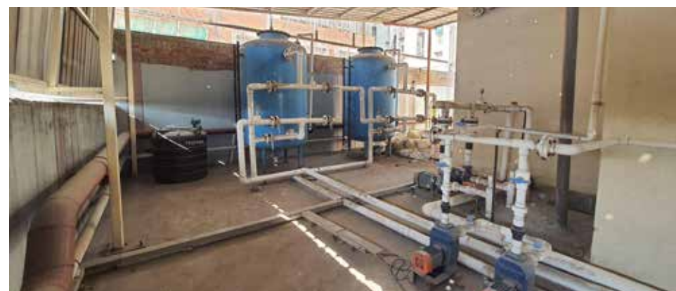
Image 12: Tertiary Sewage Treatment Plant
