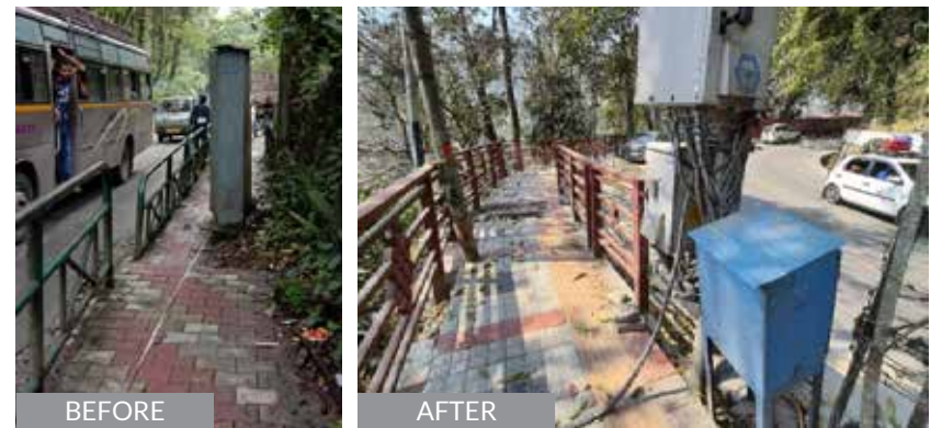
Figure 14: Shifting utility boxes before shifting (left) and after shifting (right) Source: DPR, 2018 (left) & IIT Kharagpur Survey (right)
