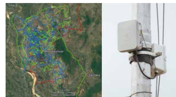
Figure 19: City-wide optical fibre network (left), Wi-Fi access points (right) (BSCL, 2022)
