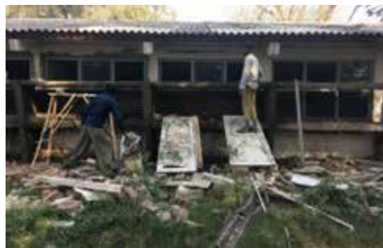
Figure 2.33: Damaged louvres being re-casted Source: Author
