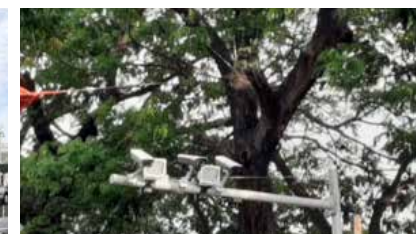
Figure 6: CCTV cameras for ITMS
