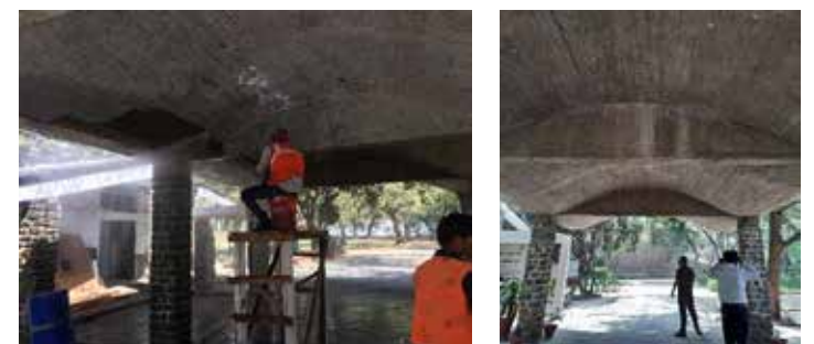
Figure 2.17: Water jetting cleaning of the exposed concrete surface being used at Le Corbusier Centre (above); Source: Ar. Deepika Gandhi Final cleaned concrete (below); Source: Author
