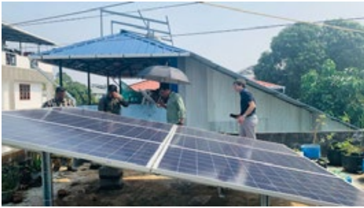
Solar Installation at a household for the Sustainable Neighbourhood project
