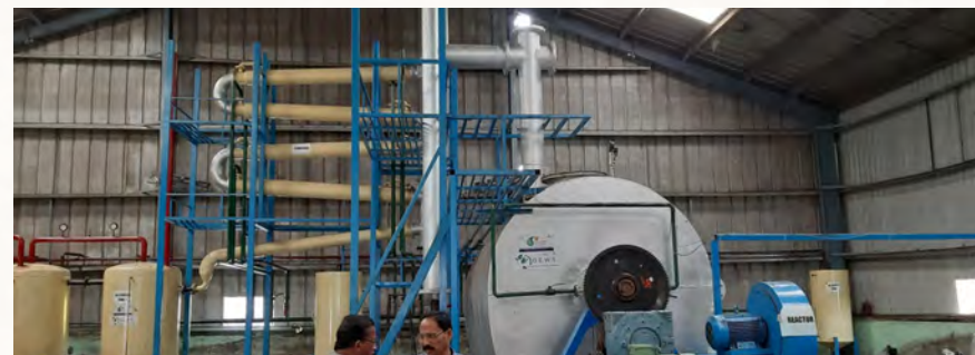
Plastic to fuel plant
