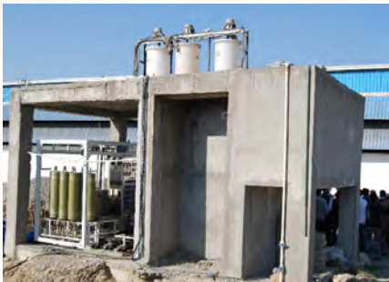
Leachate Treatment Plant
