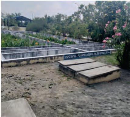
Septage passed from drying bed to Horizontal Gravel Filter
