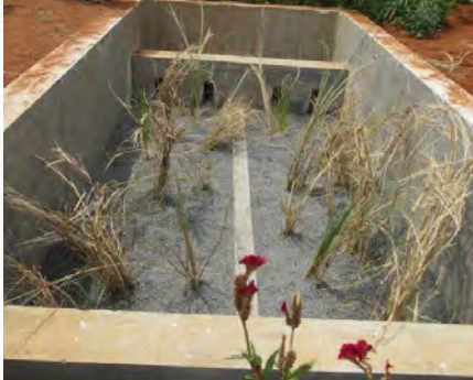
Horizontal-flow Constructed Wetland
