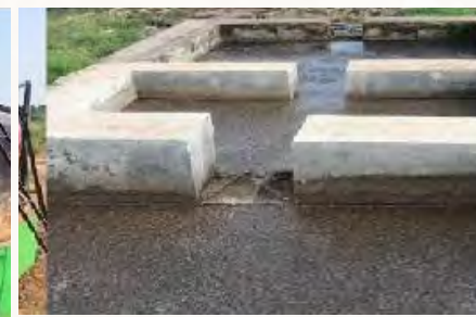
Sludge in the outlet tank
