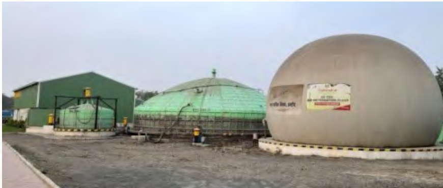
Main Digester and Balloon
