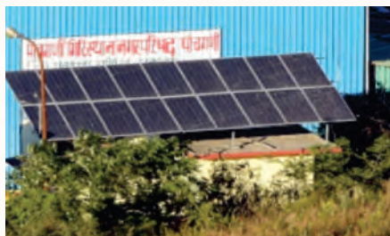
Solar panel installed at the facility
