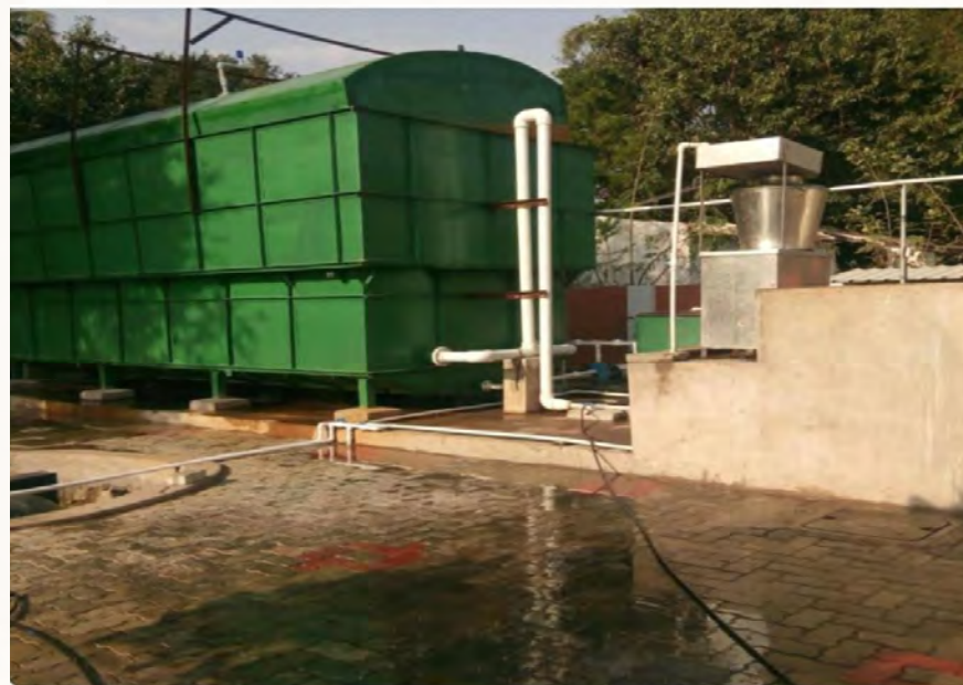
Biogas Plant at Najundapuram crematorium
