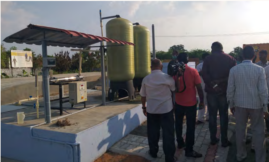
Pressure Sand Filter (PSF), Activated Carbon Filter (ACF) and UV Disinfection Unit
