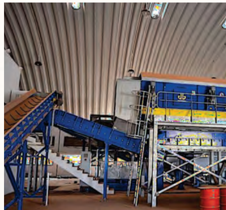
Roller screen followed by a sorting station to recover recyclables
