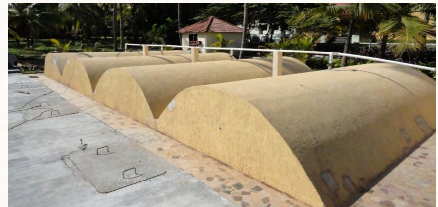
Biogas facility at Infosys Campus, Mysore
