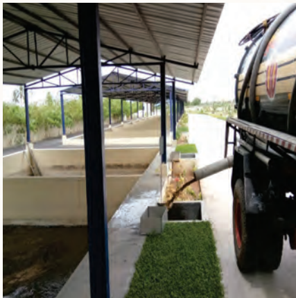
Emptying of septage into drying bed
