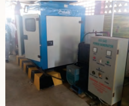
Biogas power generator
