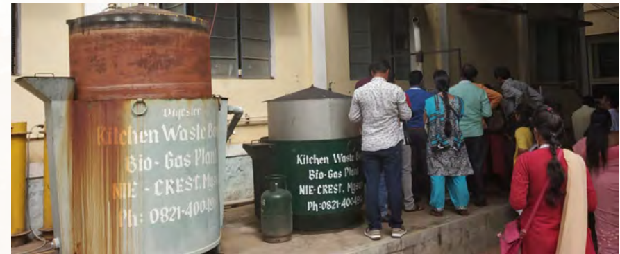
Kitchen waste based biogas plant
