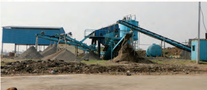
C&D waste recycling plant
