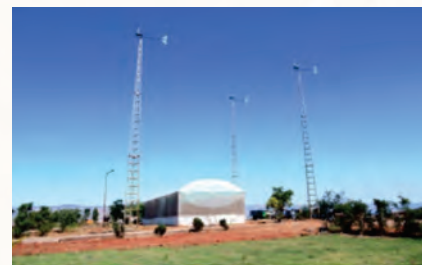
Windmills installed at the facility
