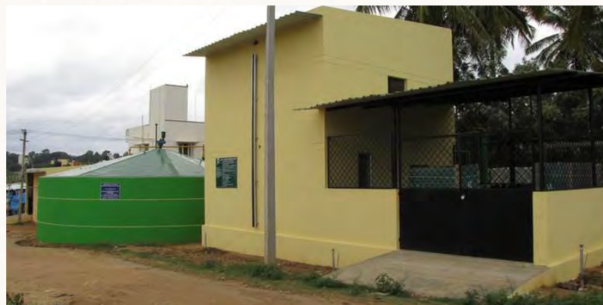
Bio Methanation Plant at Kuvempu Nagar
