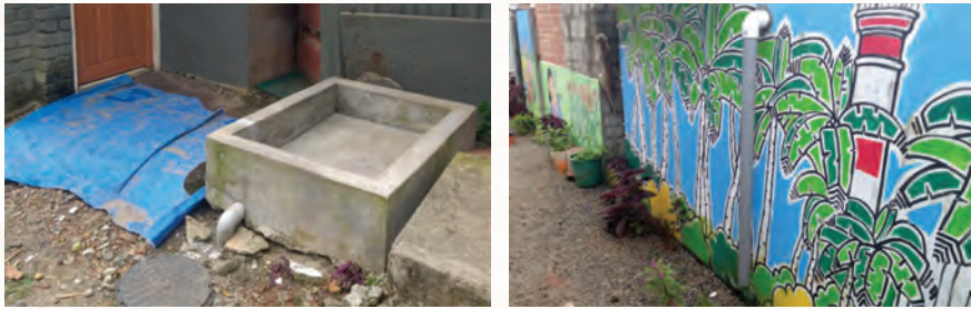
Black and Grey water pipes from households connected to common underground pipe leading to settling tank
