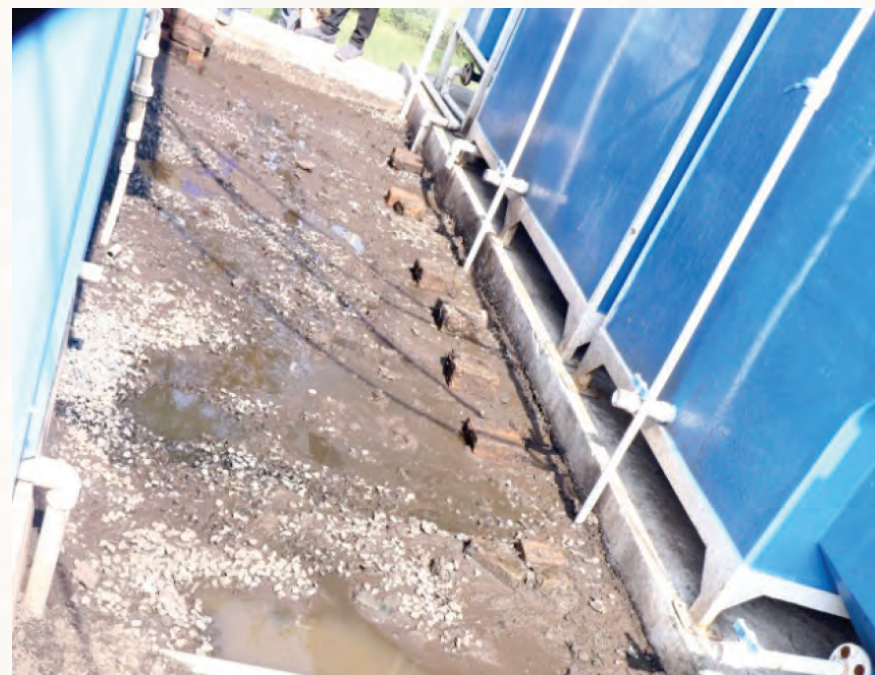
Faecal Sewage Treatment Plant based on Hyper Core Technology
