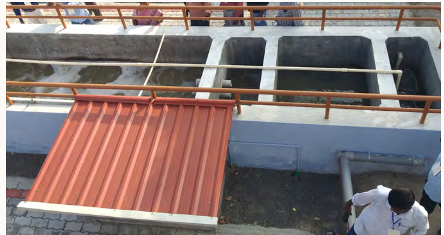
Moving Bed Biofilm Reactor
