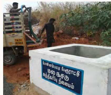
Unloading of septage into Feeding Tank
