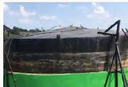
Floating dome Digester
