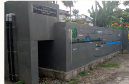
Planted gravel filter
