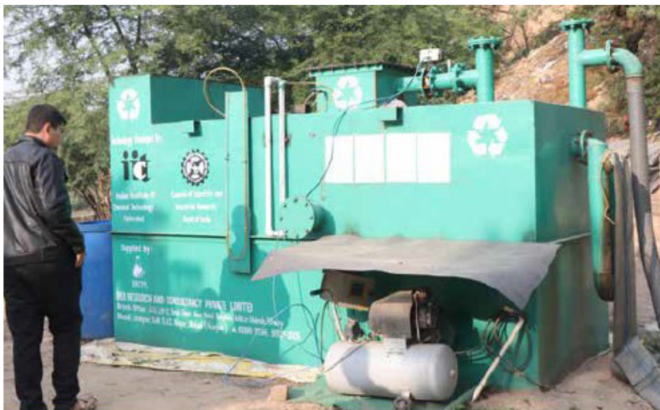
Figure 4.49: Biogas plant at Chandigarh
