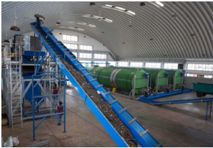
Figure 4.75: In vessel composting drums, compost screens
