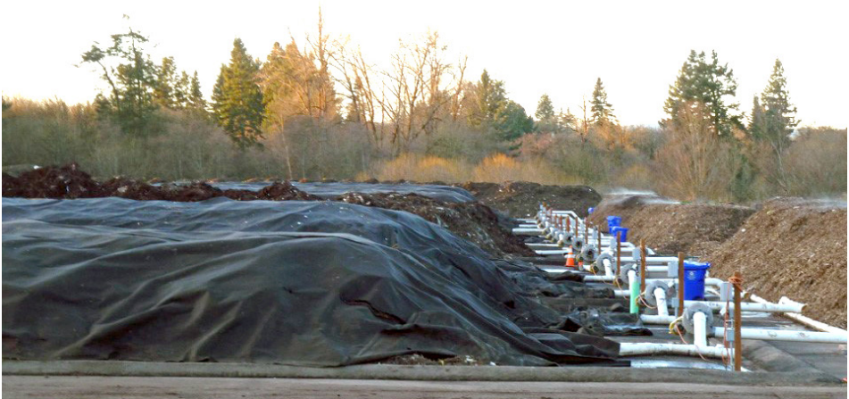
Figure 4.73: Covered Aerated Static Pile Composting at Gajuwaka
