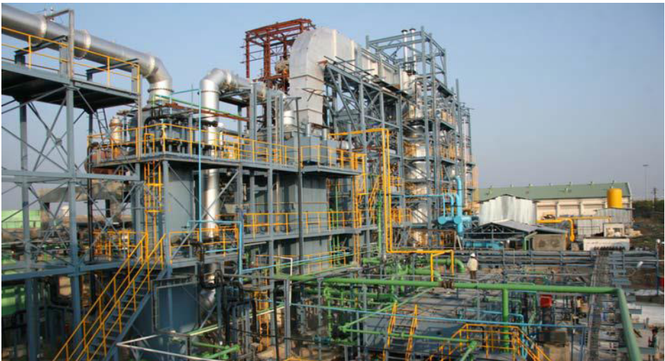
Figure 4.81: Plasma Gasification Facility
