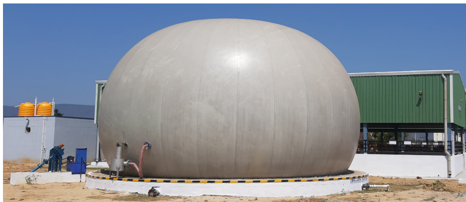
Figure 4.42: Biomethanation plant at Thukivakam
