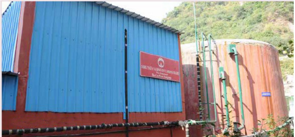
Figure 4.46: Biogas plant at Banganga
