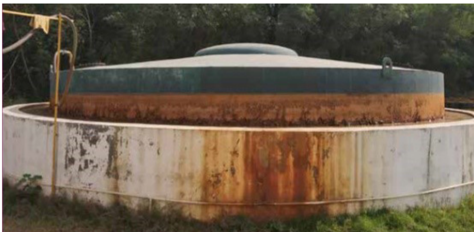
Figure 4.45: Biomethanation-cum- electricity plant at Chandigarh
