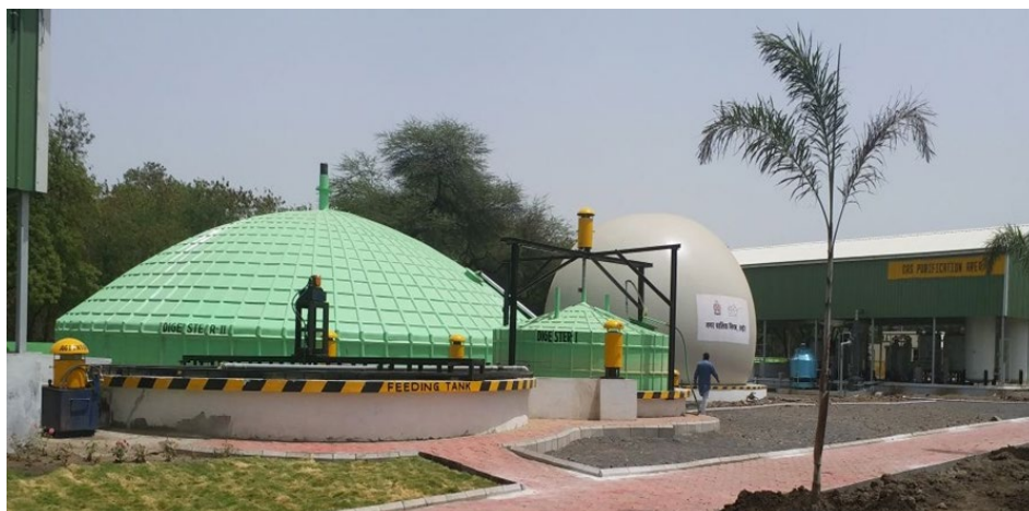
Figure 15: A view of 20 TPD Bio-methanation Plant at Indore
