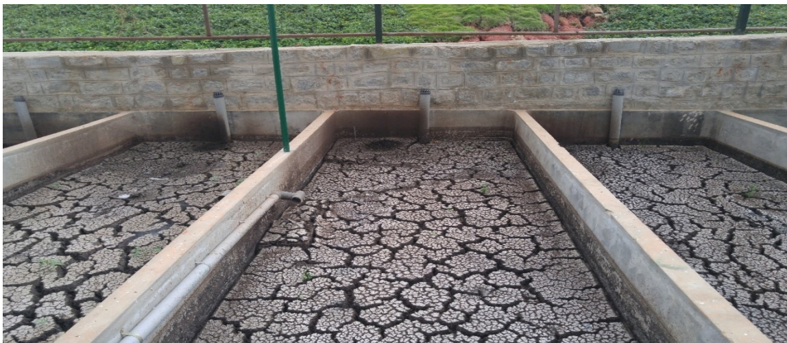
Figure 43: Sludge Drying Bed
