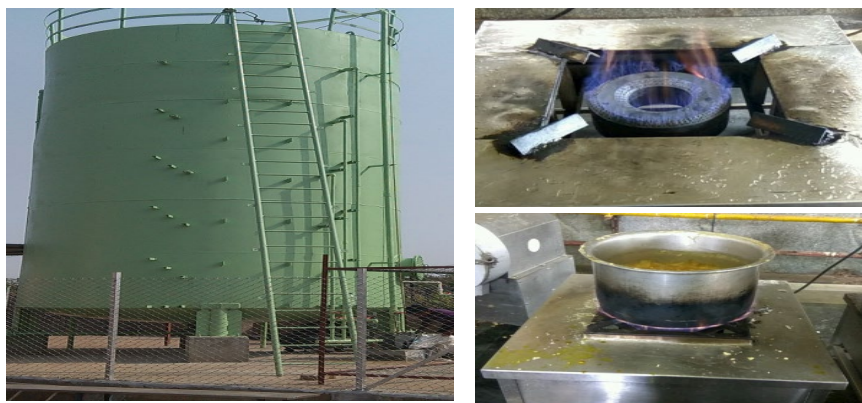
Figure 16: High Rate Biomethanation Plant at Toranagallu (Bellary), Karnataka
