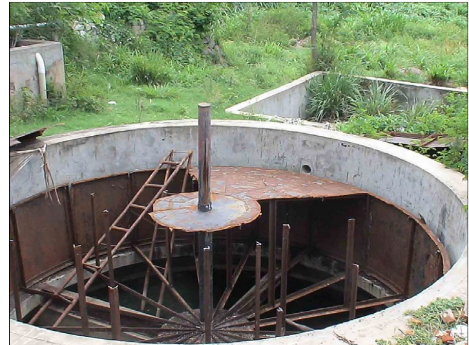
Biogas plant at Mysuru Zoo
