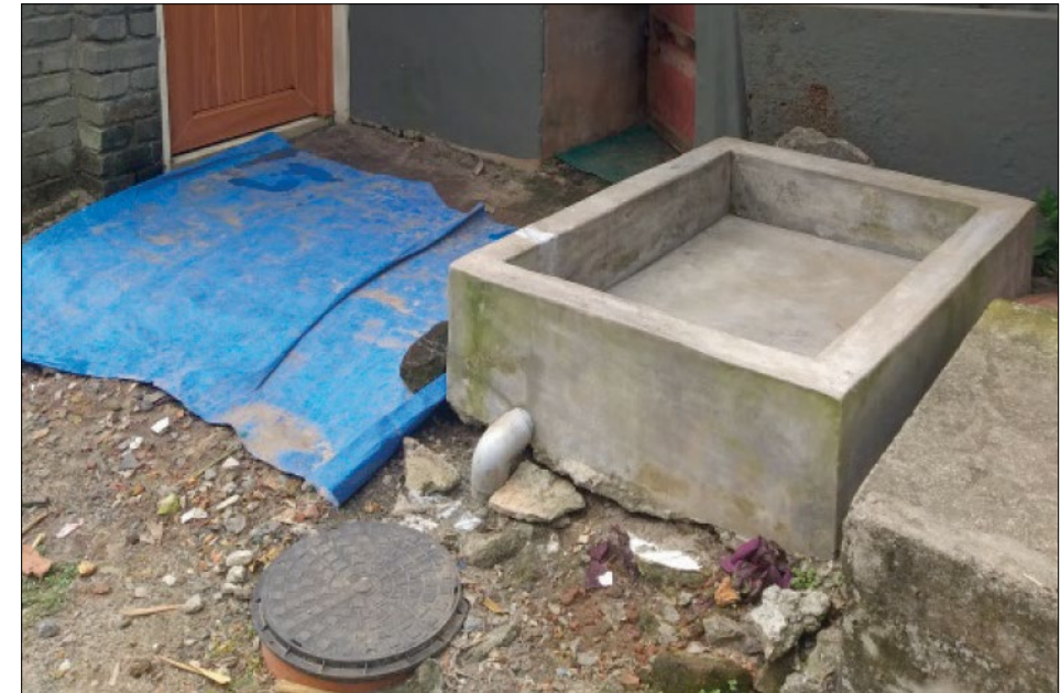
Black and grey water pipes from households connected to common underground pipe leading to settling tank
