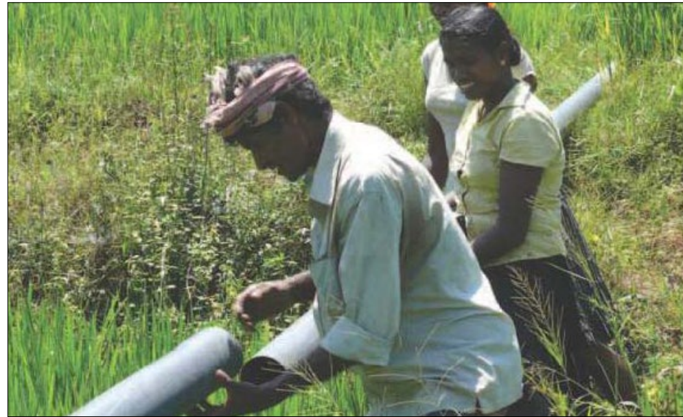
Installation of (bio)diesel-operated water pump Source: ENERGIA report 'Mainstreaming Gender in Energy Projects A Practical Handbook'
