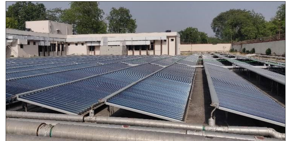
A solar thermal field comprising 525 solar thermal collectors
