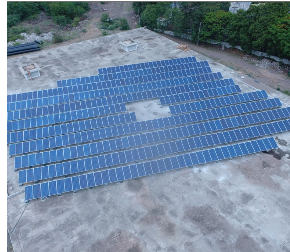
145kWp grid-connected Solar PV system as part of the project
