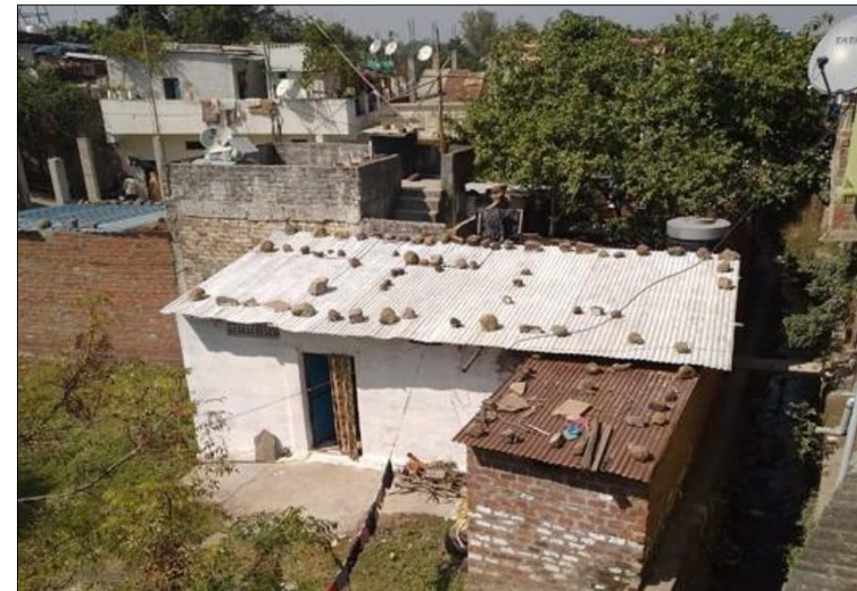
Solar reflective paint on the roof keeps indoor temperatures 1.5 to 5°C lower than conventional roofs
