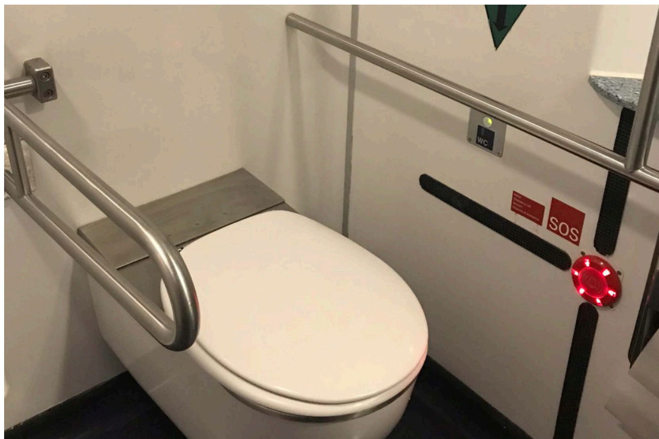
Image 28 Emergency Warning Alarm Switch near Accessible Toilet Source: (Ministry of Housing and Urban Affairs, Government of India, 2021)
