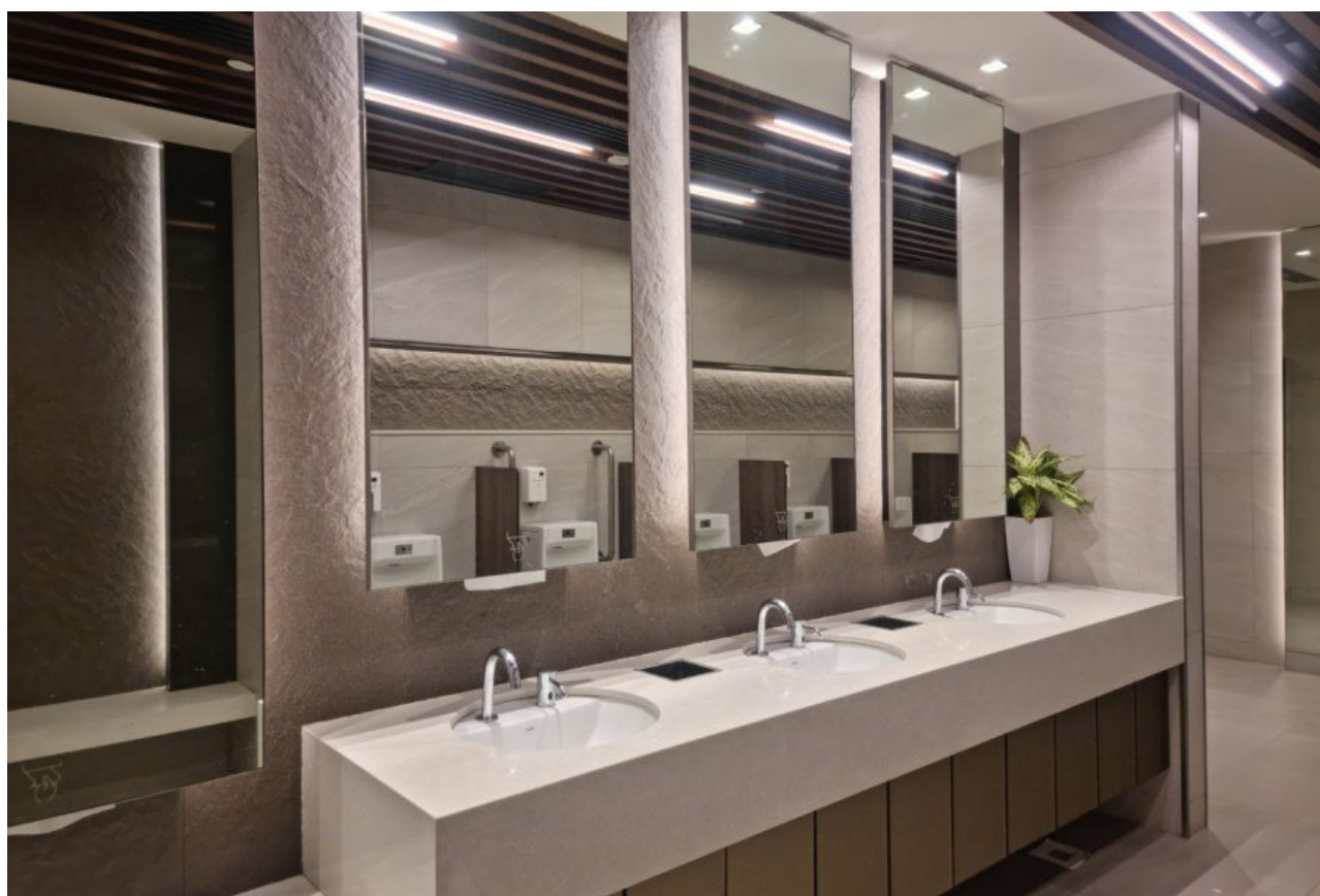
Image 9 Vanity top-cum wash basins
