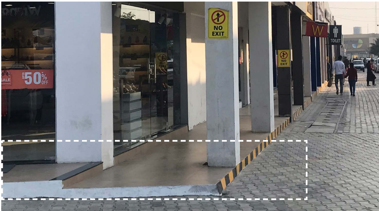
Image 2.15 Improper edge detailing of level change
