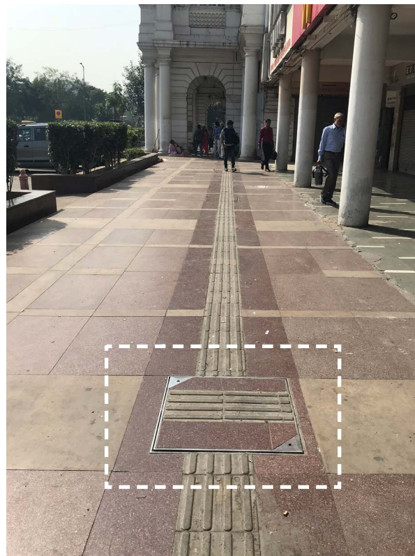
Image 2.20 Inconsistent laying of tactile guiding tiles
