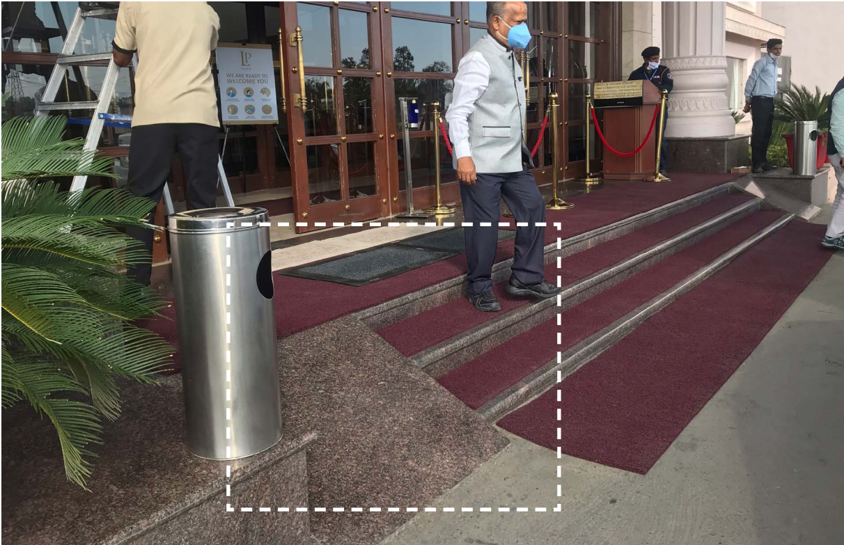
Image 2.7 Improper ramp gradient and slippery floor finish
