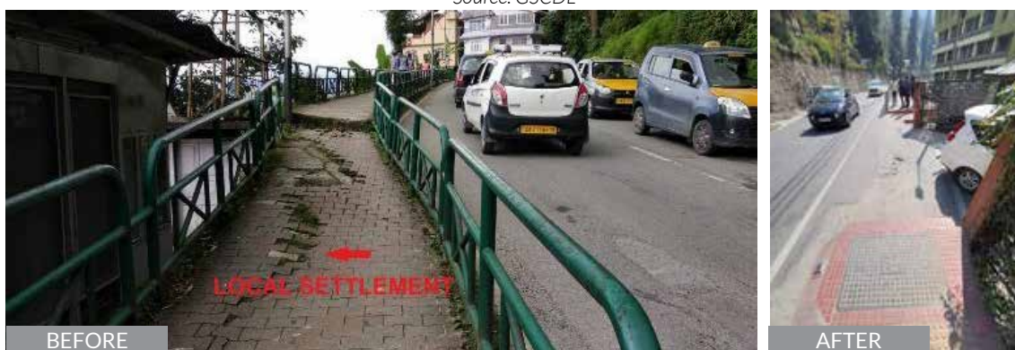
Figure 13: Surface of footpath Source: DPR, 2018 (left) & IIT Kharagpur Survey (right)
