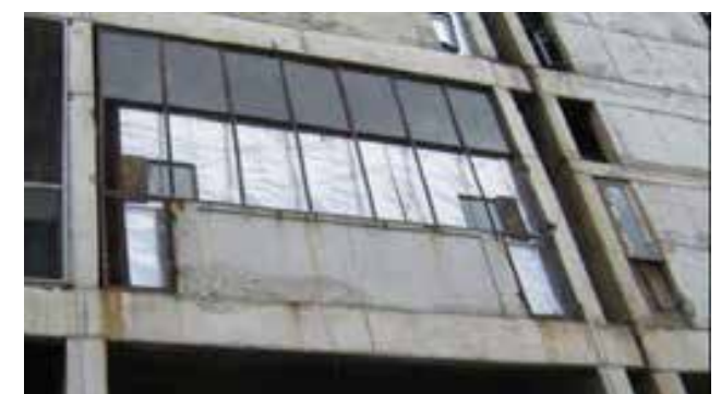
Figure 2.6: Extension in the original veranda Source: Chandigarh Heritage Report by Heritage Conservation Committee of Chandigarh
