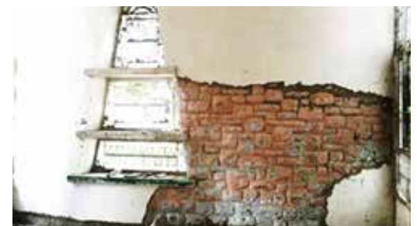
Figure 2.28: Plaster chiselled out to reveal original rubble masonry wall Source: Ar. Deepika Gandhi
