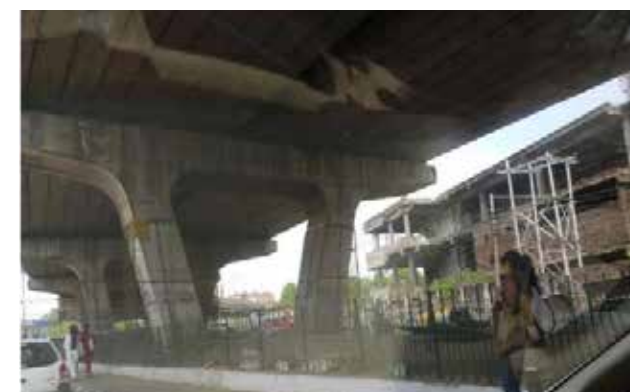
Fig 7: Area under Flyover DC Chowk and Jewel Chowk [before intervention]
