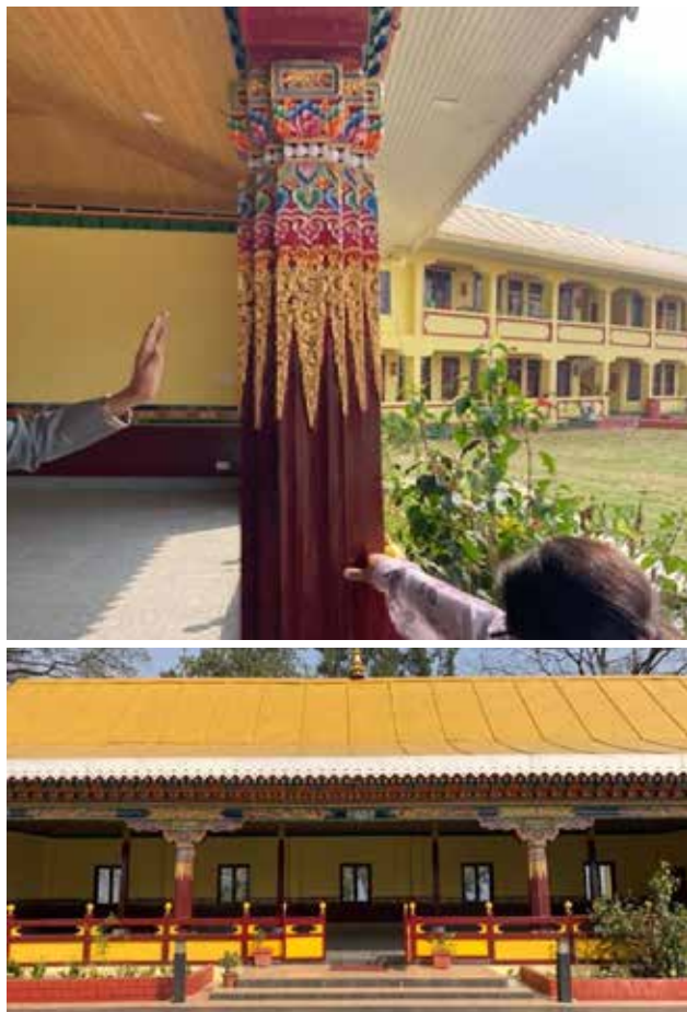
Figure 14: One of the older columns in the Yabring restored (L), the restored Yabring (R)
