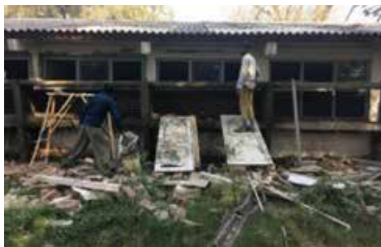
Figure 2.33: Damaged louvres being re-casted Source: Author
