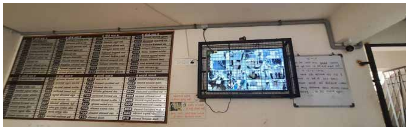
Image 9: Boards with campus name, owner name ad flat no and security monitors at the entrance of every building
