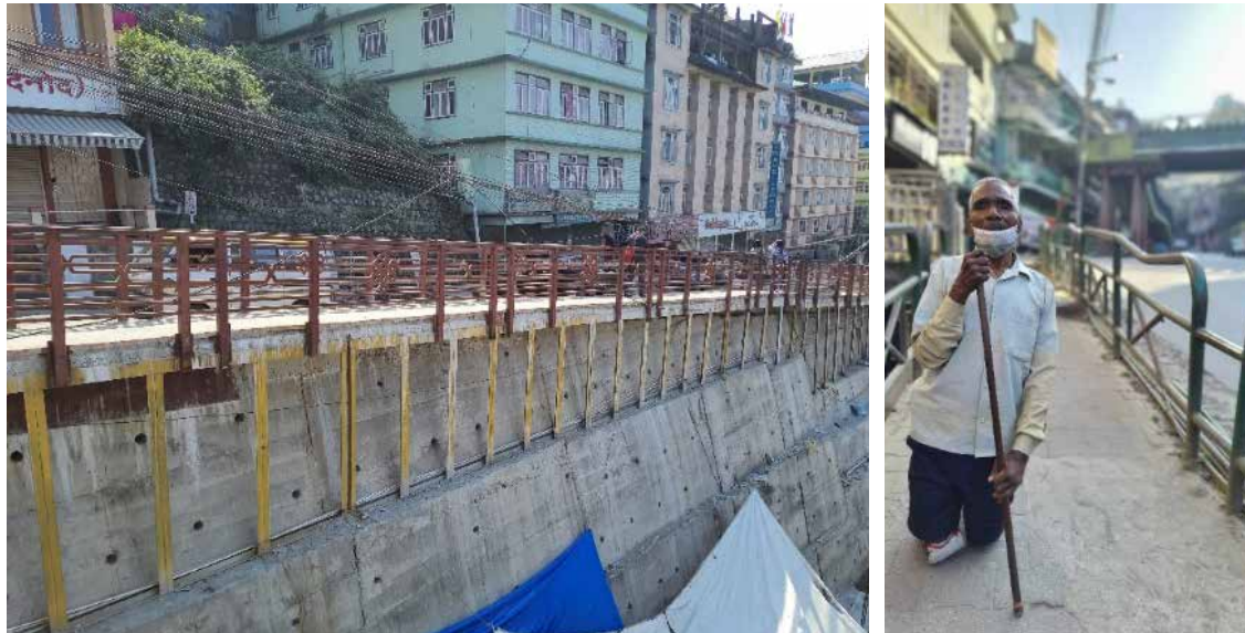
Figure 17: Overhanging footpaths: Sisagolai (left) & Specially-abled user on the footpath (right) Source: IIT Kharagpur Survey
