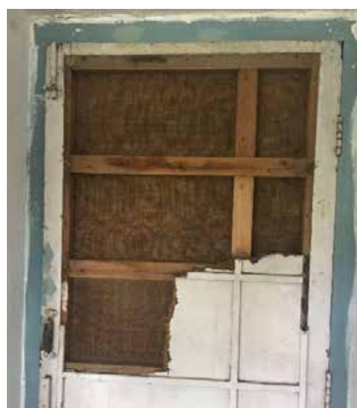
Figure 2.11: Broken and damaged door made up of cardboard and jute for passive cooling at Le Corbusier Centre; source- Ar. Deepika Gandhi
