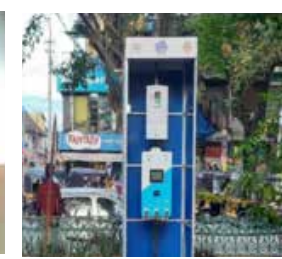
Figure 4: EV charging station
