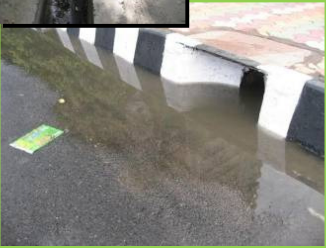
Overflowing Storm Water Inlet, ITO
