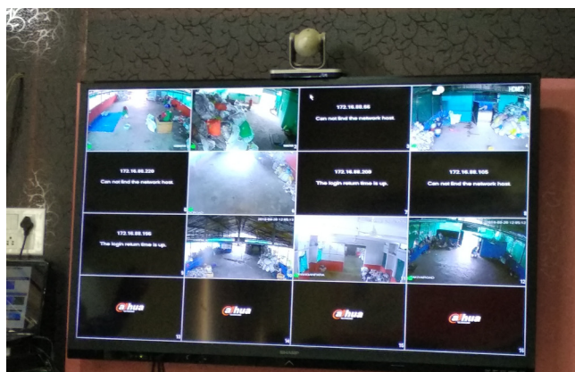
Figure 29- Central control room to monitor real time activities
