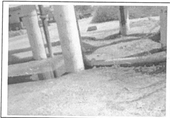
Photograph 51: Leakage in the water supply main at the OHSR
