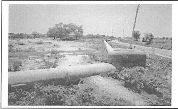
Photograph 14: Inlet Pipe for carrying raw water from source
