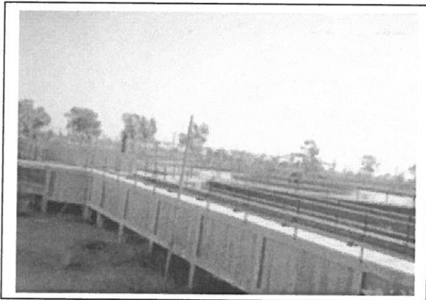
Photographs 54: Water treatment plant at Kekri – Clarifier
