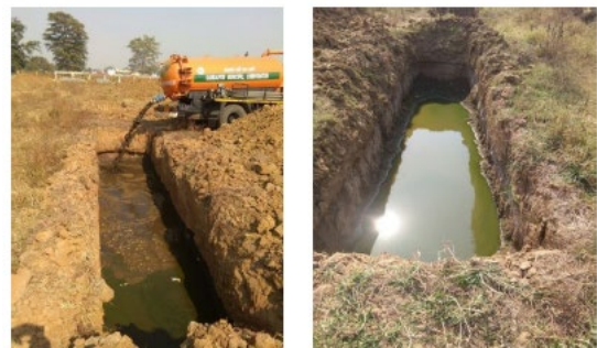
Figure 36 – Deep row entrenchment
