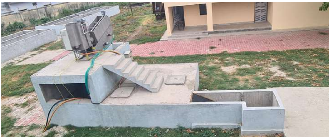
Image 10: Co-treatment unit for Faecal Sludge/Septage at STP
